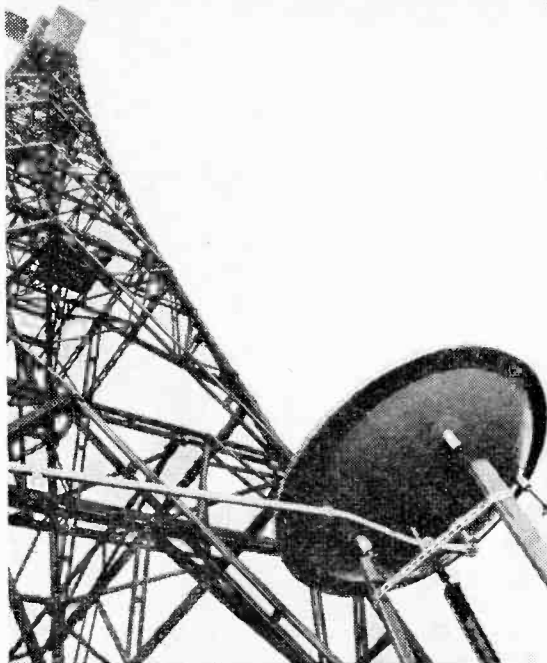
Plane passive reflector on mast reflects to next repeater beam from aerial at ground level.
